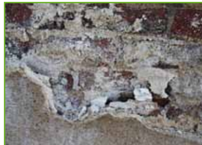
Typical damage through salt efflorescence.
