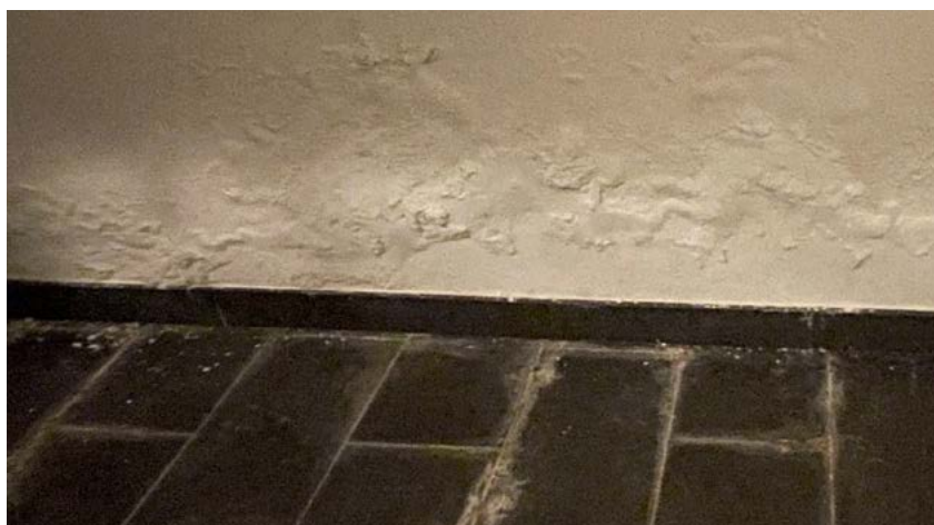
Typical Signs of Rising Damp
